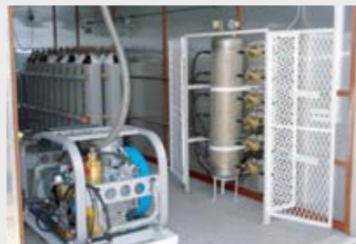
20ft Containerized B.A. Cascade System
